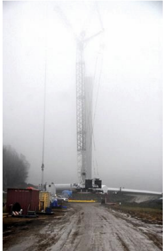
The base of turbine 1A in Cohocton disappears into the clouds during its construction Monday afternoon.
