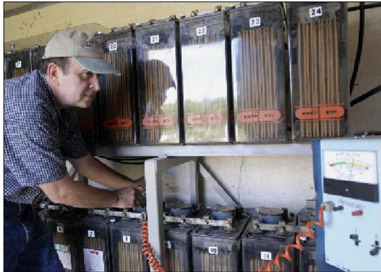
Yuri Odeychuk, 48, of Orleans County checks the batteries that store the power generated by his wind turbine. The Hamlin Town Board put a one-year moratorium on wind turbines while it researches regulation. A large-scale turbine project also is emerging in six Wayne County towns.
